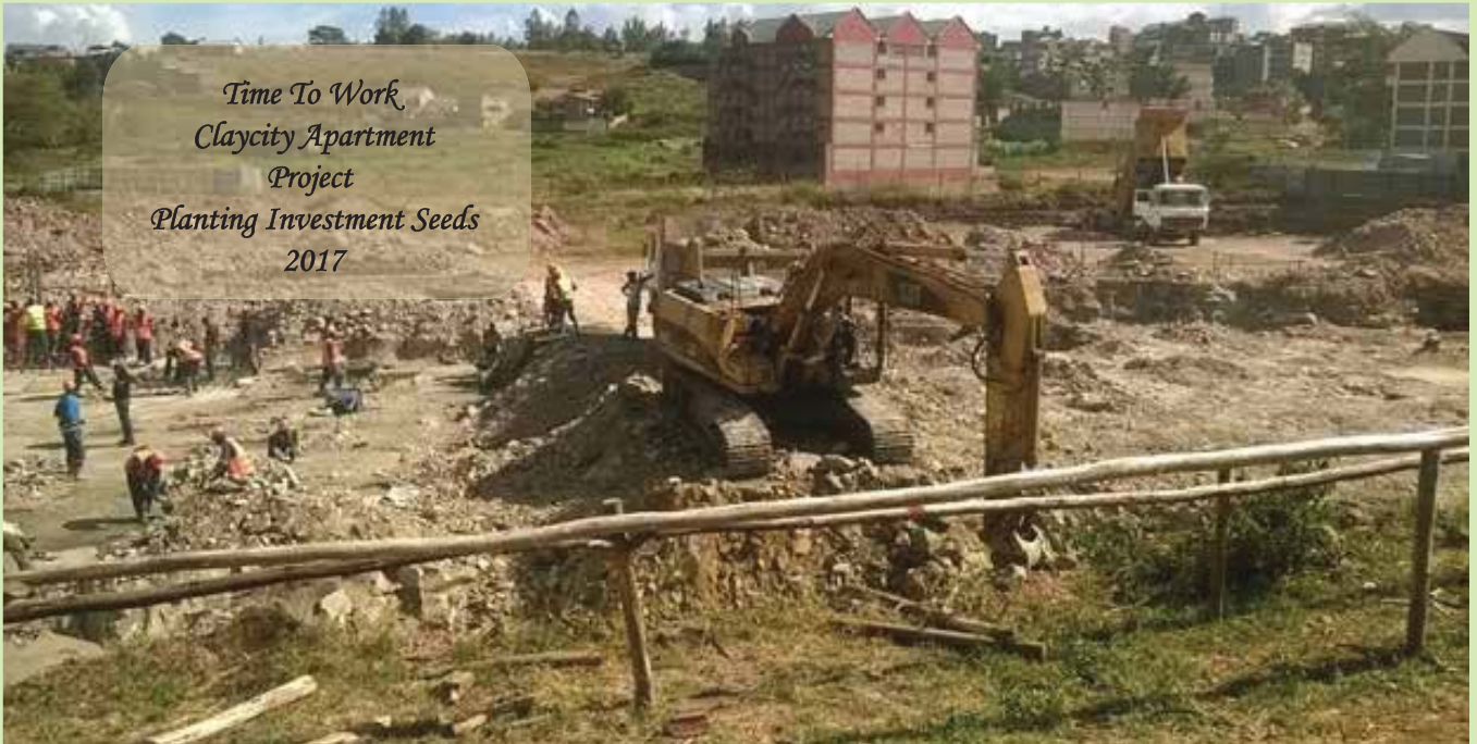
ClayCity apartments project, construction work on site by contractor Jinsing Enterprises Co. Ltd in February 2017
